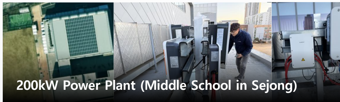
Sungrow 200kW-class solar inverters (4 units)
