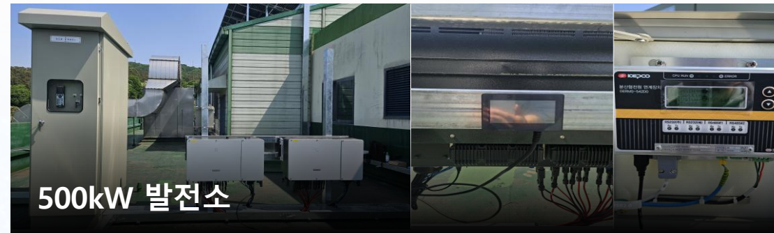
Sungrow 100kW-class solar inverters (5 units)
